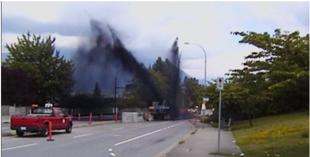
Shawn Soucy photo. In Burnaby, at 12:31 pm, July 24, 2007, a contractor ruptured the Kinder Morgan high pressure oil pipeline between Burnaby Mt. and the marine terminal. 11 homes were covered in oil, 250 residents were evacuated, 250,000 litres of oil were spilled into Burnaby Inlet, with 210,000 recovered. The clean up cost 15-17 million dollars.
